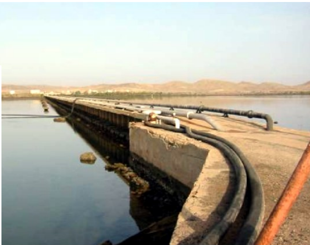
Above: Part of the new Hirgigo fuel jetty undergoing construction in Massawa
